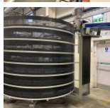
18166 Ambaflex 50 mt drytower 50 meter belts Entrance from the left under Exit to the right
